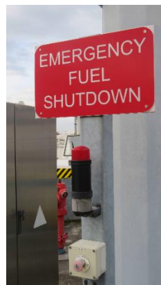
Figures 7 and 8. Emergency stop buttons
